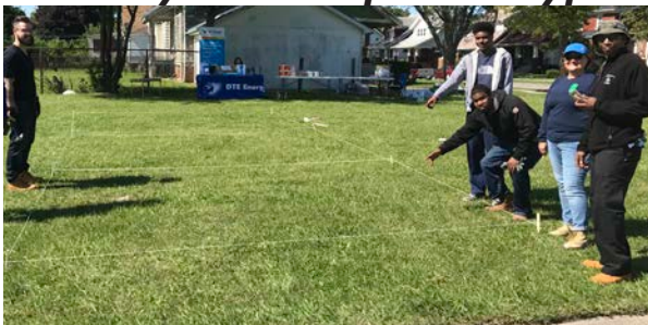
IS@H and studio[Ci] pose while pointing at the staking of the new HNZE Canopy
